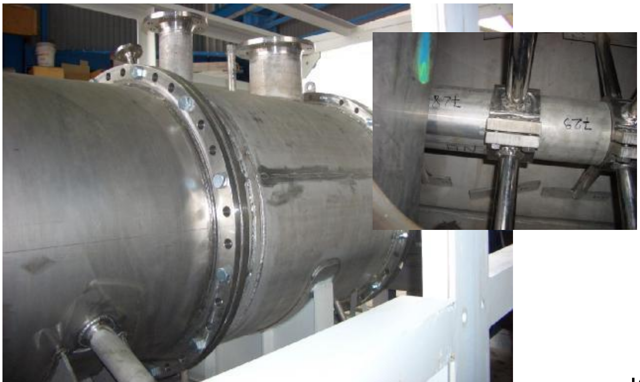
Picture 3: Module 1 – entry with heating zone for fuels (LMSV)
